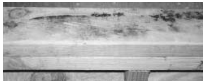
Fig. 3: Mold on lumber
